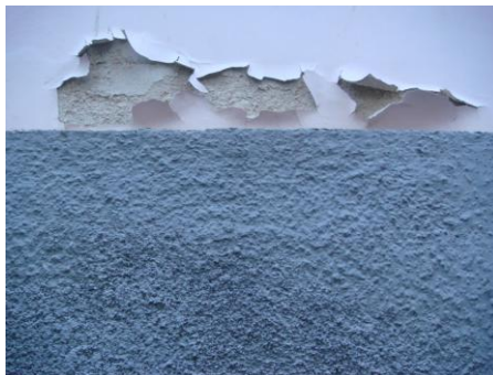
Fig. 3 The deterioration of cement plaster at House of Rui Barbosa's surfaces-detail
