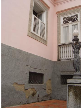
Fig. 2 The deterioration of cement plaster at Casa de Rui Barbosa Museum's surfaces
