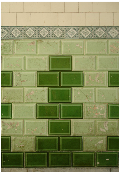
Vista geral do painel
